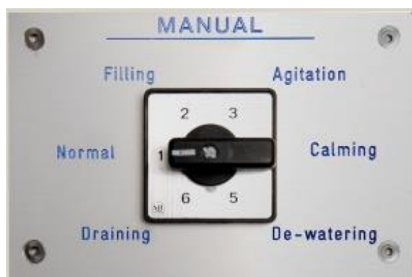
Manual control via selector switch
