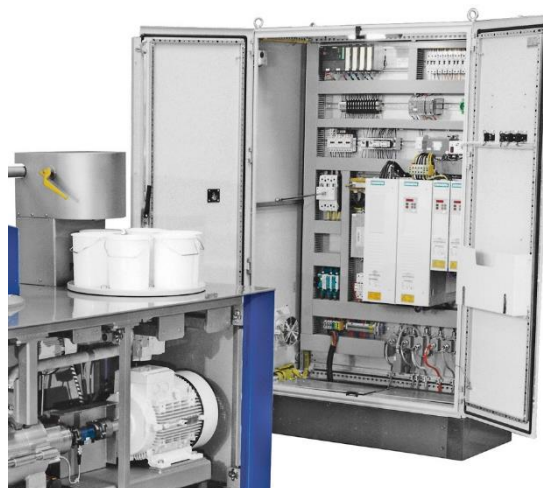
Separate control cabinet
